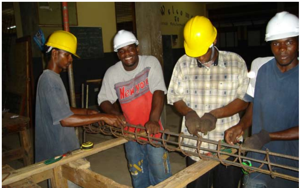
CYEP students learn new construction skills in training class held in St. Patrick Parish, Grenada.
